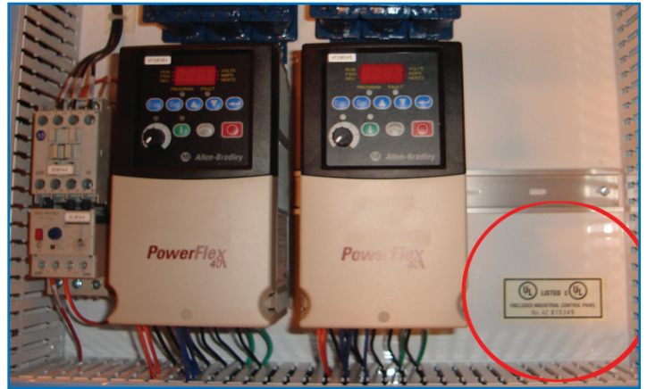
U.L. sticker is shown inside an electrical panel.
