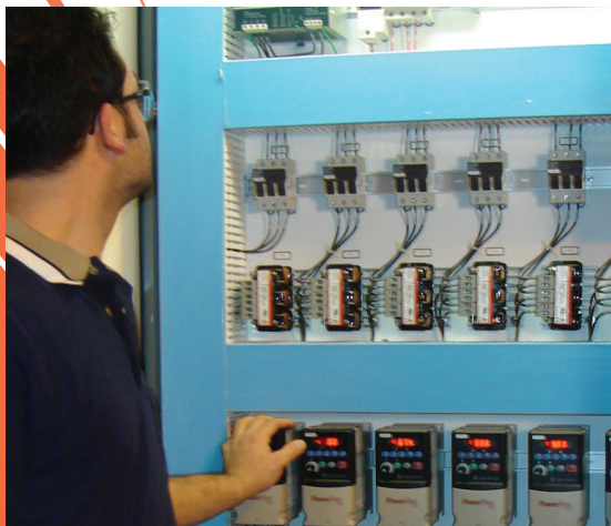
Electrical controls manager verifies panel operation.
