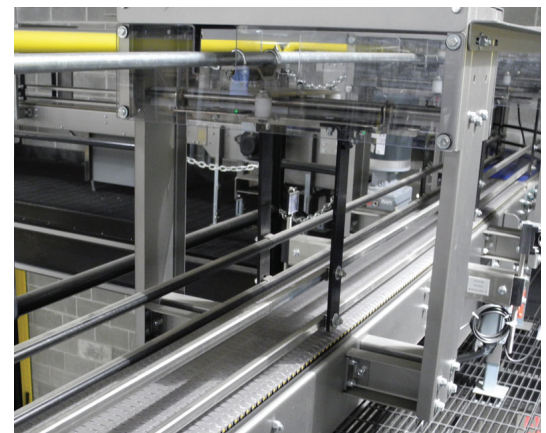
Dual lane automatic guide rail system utilizing electric actuated cylinders.
